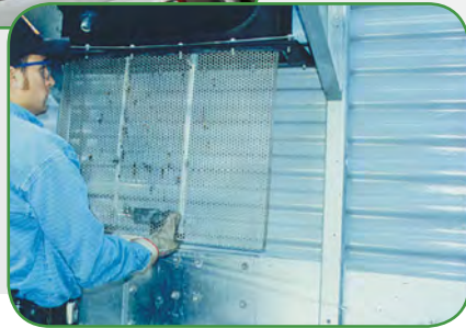
Inlet strainer inspection for Series 3000
